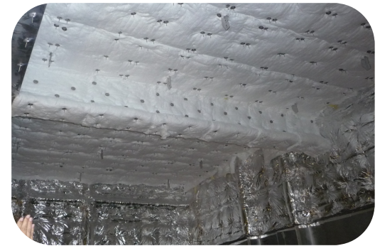
10,000 m 2 FireMaster Marine Plus Blanket installed in 2011 for one hour fire protection of external and internal structure
